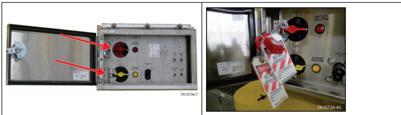
Battery isolation switch in OFF position with locks in place
